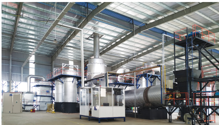
▲ The Incinerators of the Facility, two of the largest in HCMC with a capacity of 48 tons a day
